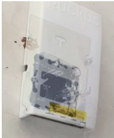
FIGURE 8: WALL MOUNTED ACCESS POINT
