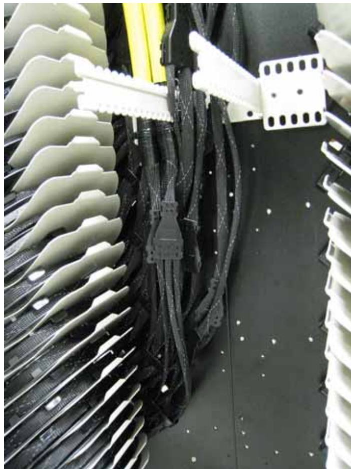
Figure 15. IFC and OSP Cables Routed Into Splice Shelves
