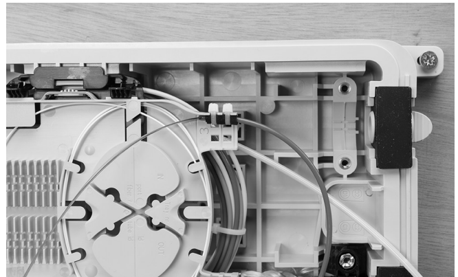
3.3.18 Remove the excess tube and secure the end of the tube using cable ties as shown. Clean the fiber.
